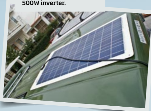
75W solar panel by Conergy provides 220V electricity through an auxiliary 45A dry type battery and a 500W inverter.
